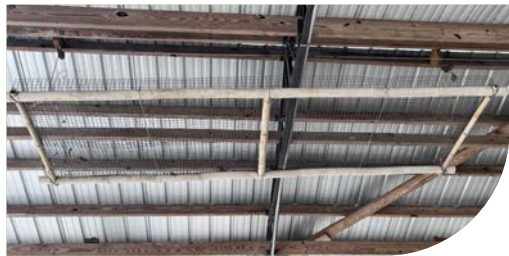
A rack suspended near a metal roof.
