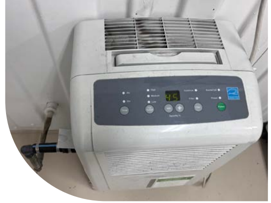
A dehumidifier with drain line.
